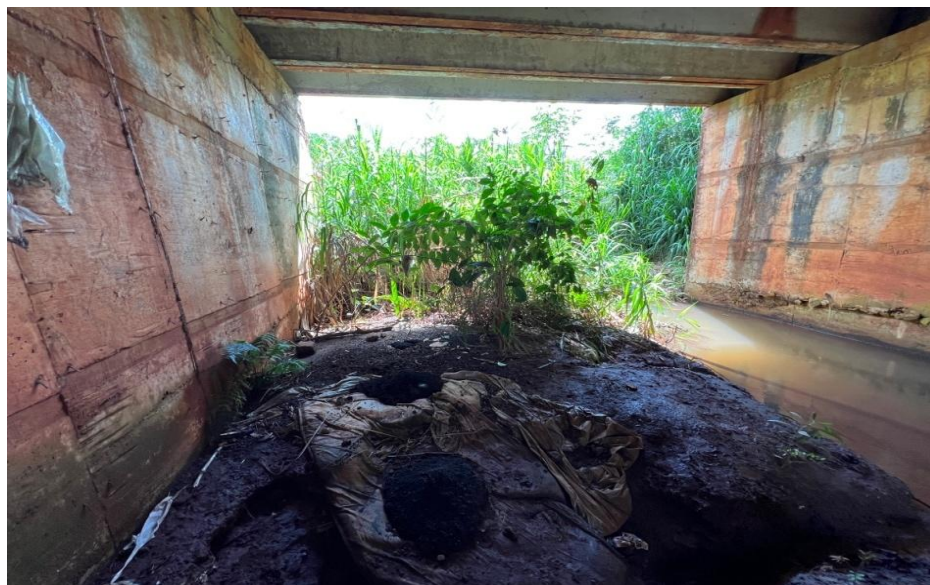
Figure 6 - Trash on the stream banks under the bridge.
